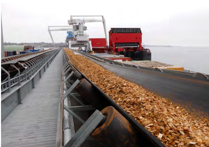
2 x 1400 m 3 /h Conveyors upstream screening building
